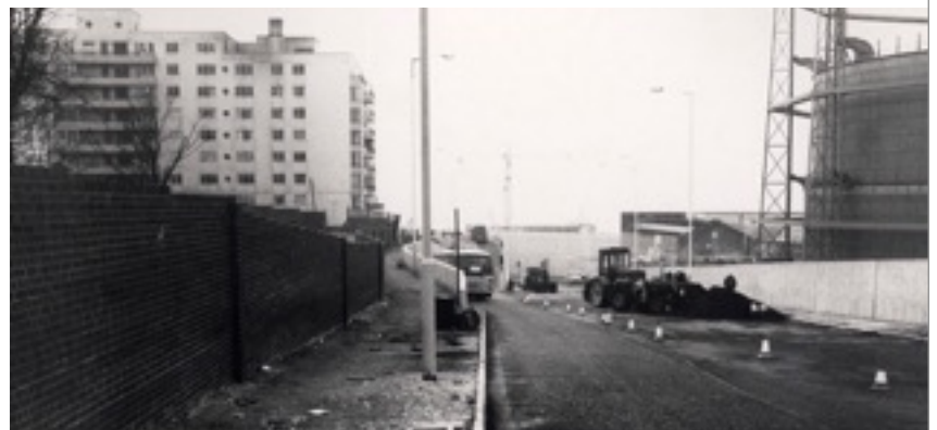
above : an earlier view of MG during construction of access to the new marina
